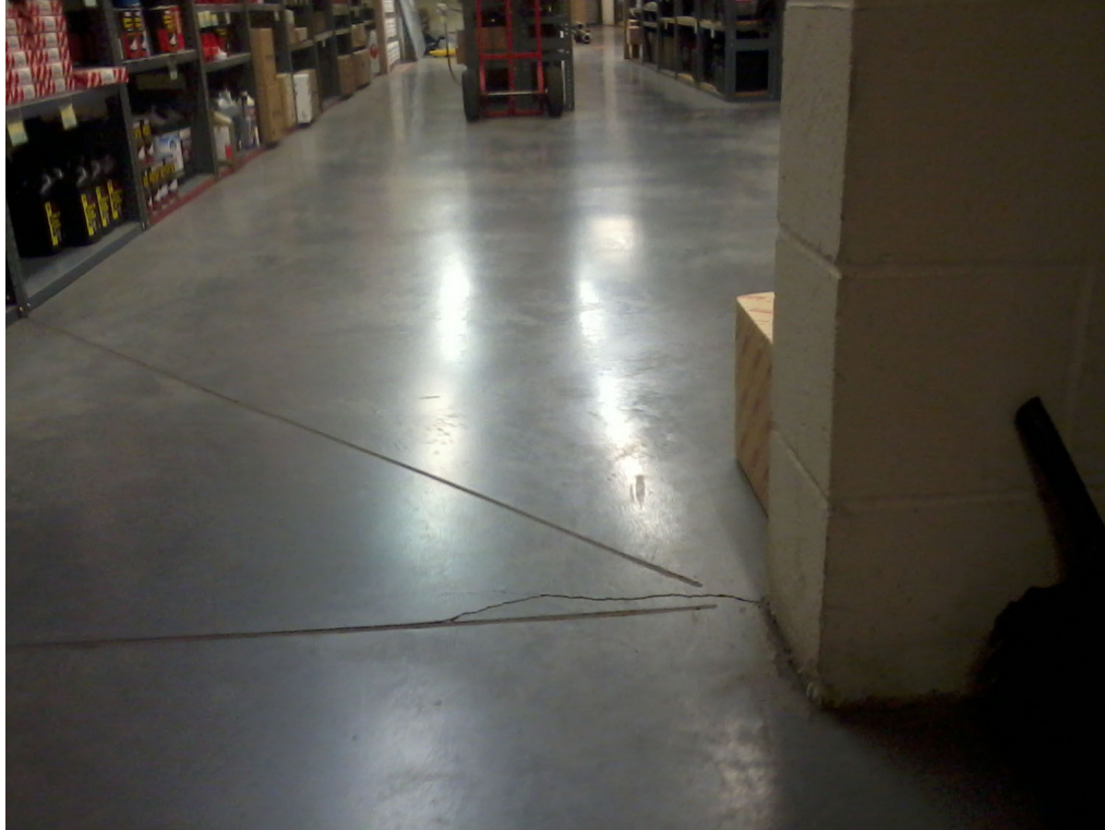
Figure 11 Only Floor Crack in Entire Concrete Slab
